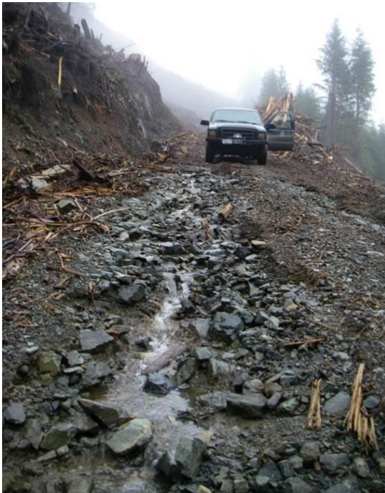
Figure 13: Roads can intercept and redirect water, concentrate flows and be a source of fine sediment that can affect aquatic ecosystems. Images: R.G. Pike.
